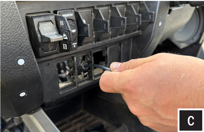
C. Fish thru the LCD Touch Button Controller cable into the dash cavity.
